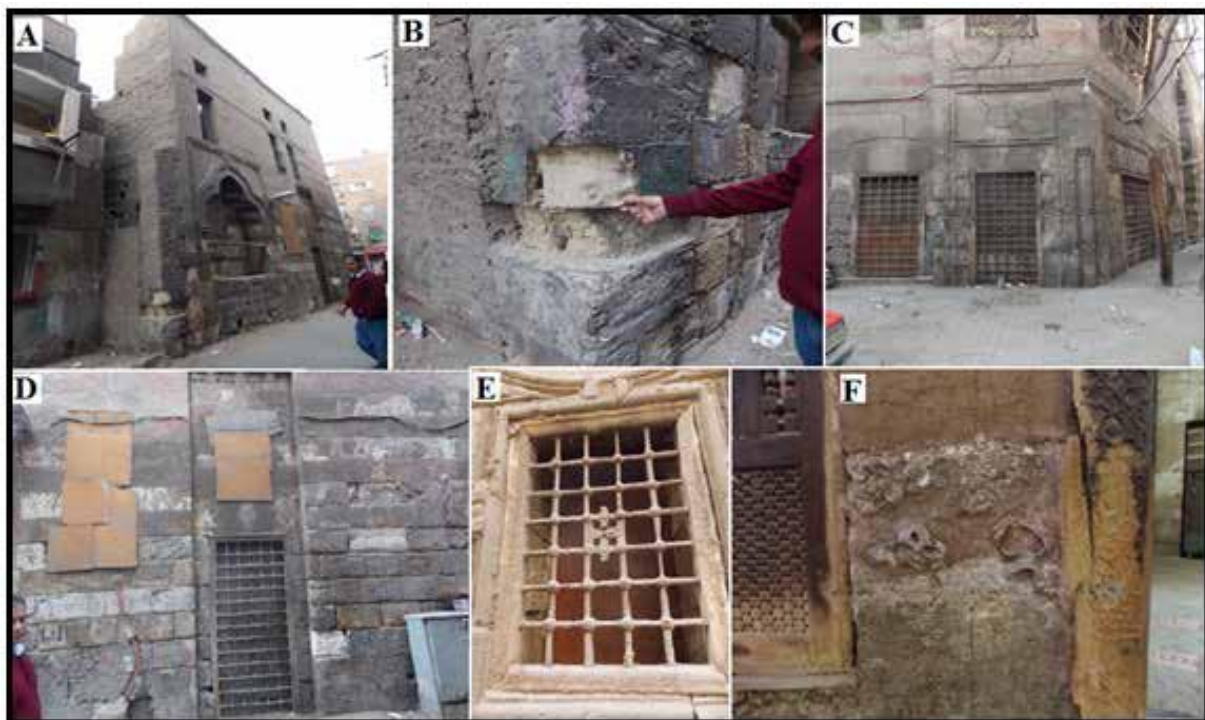
Picture 7: (A) illustrates the infringement of modern building around the School - (B) illustrates the loss of some parts of the stone courses - (C) illustrates the low level of the court as opposed to the street level - (D and E) illustrate the extent of rust of the iron windows and their coverage with a black layer - (F) illustrates the deterioration of wood due to moisture and salts. (Picture by the researcher)
